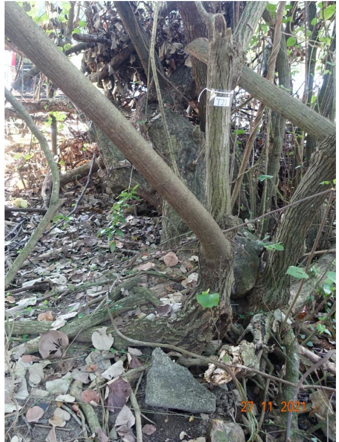
T21 LOWER TRUNK AND GROUND CONDITION - FELL
